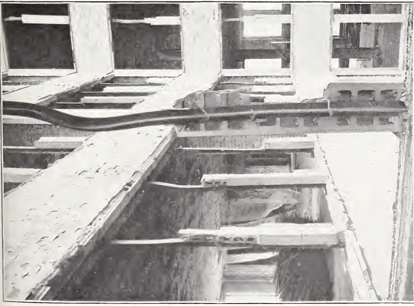
1. SPALLING OF ENAMELED BRICK IN LIGHT WELL, AND FAILURE OF FIREPROOFING OF WINDOW-FRAME SEPARATORS, MERCHANTS' EXCHANGE BUILDING, SAN FRANCISCO. Photograph by Richard L. Humphrey.
